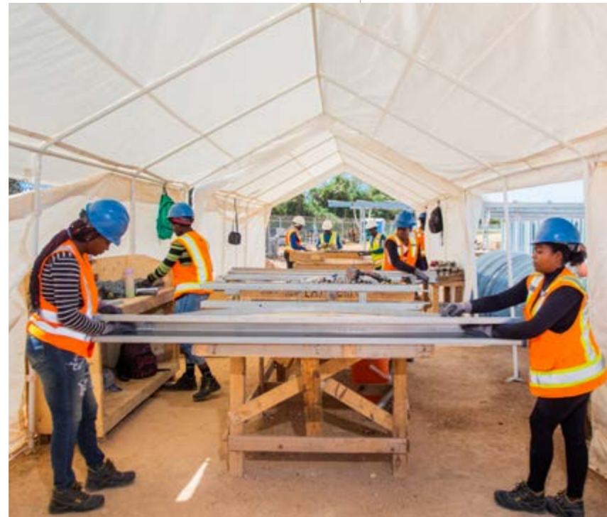
Dominican women working on the assembly of the photovoltaic structures at Ecoener's facilities in the Dominican Republic.
