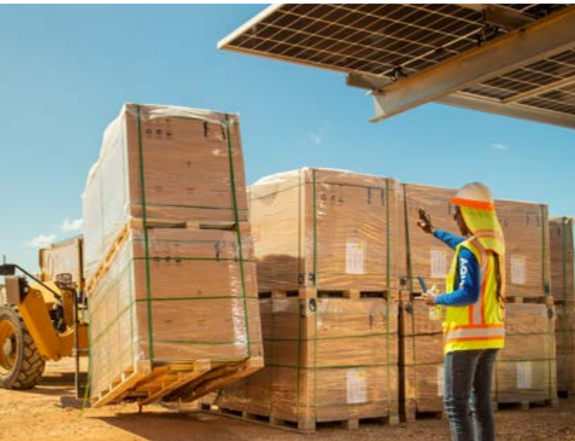
Loading and unloading work in the construction of the photovoltaic facilities in the Dominican Republic.
