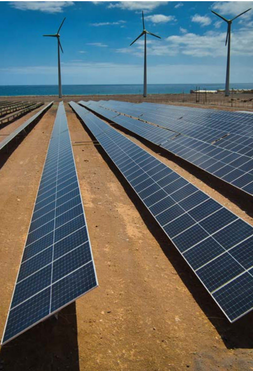
Arcos del Coronadero wind farm and Corral de Espino photovoltaic solar plant (San Bartolomé de Tirajana, Gran Canaria, Spain).
