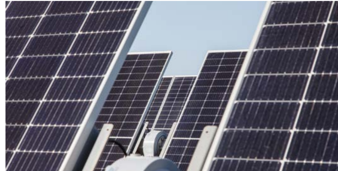
Detail of the photovoltaic panels installed in Gran Canaria.
